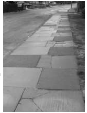
Broken pavement in Moor Park Rd
